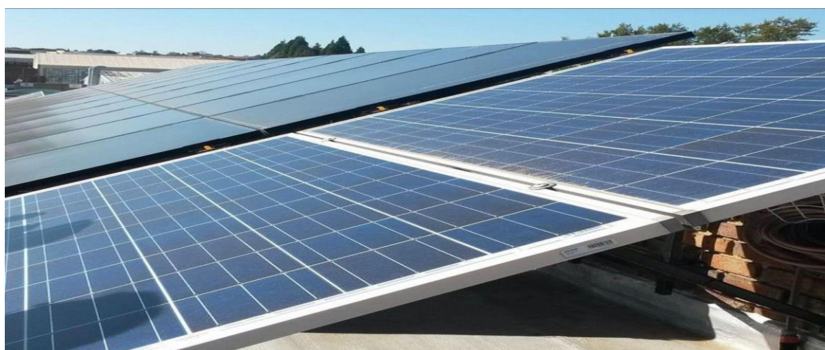
Ha Ramarothole Solar Plant Mafeteng District 70MWh solar power plant. Phase 1 (30MW)
